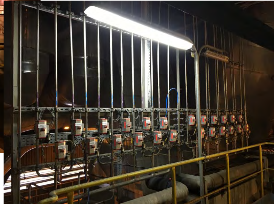
Valve Station for Injector Control
